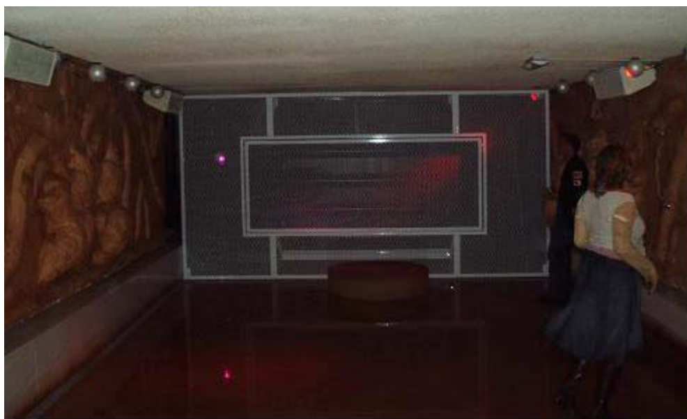
Figure 13: metal air distribution grille at the end of the dance floor.
